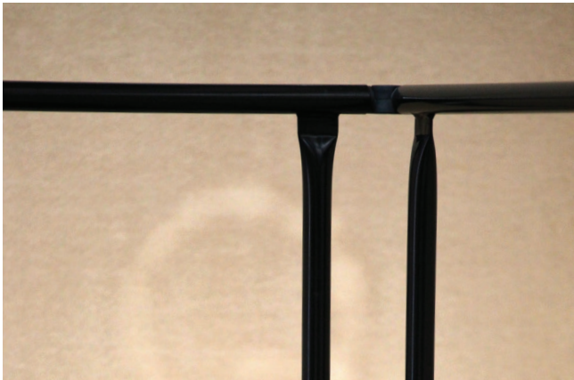
Last Hand Rails to be joined are the Top Landing 1.8m and 1.5m Hand Rail - use the Corner Joiner
